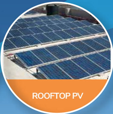
ROOFTOP PV DOUBLING AS SOLAR SHADING
